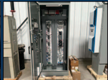
2024 ALLEN BRADLEY STARTER CABINET
