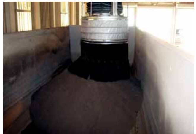
Fig. 2 & 3: Combined loading system with pneumatically operated shutter cone for loading of dolomite in closed silo trucks or open dumps. The customer's target was a drastic minimization of dust emission during the loading process. After comparing different concepts, the customer decided on this Muhr concept. The specialty of this system is the dust-free loading with both closed as well as open loading.
